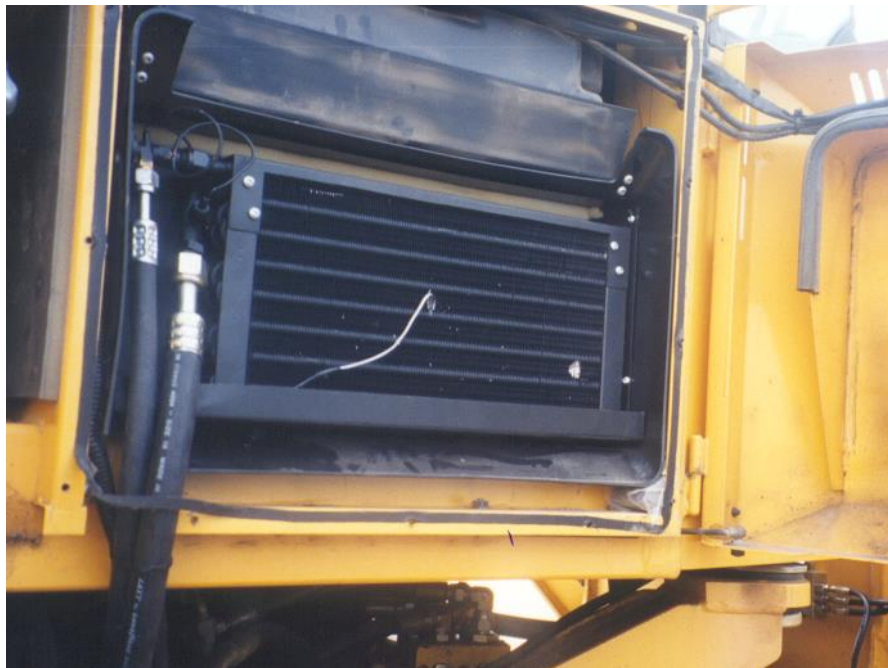
End view of evaporator assembly in place.
